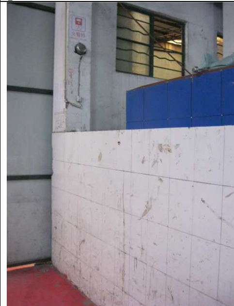
[Fire alarm button installed too high]
